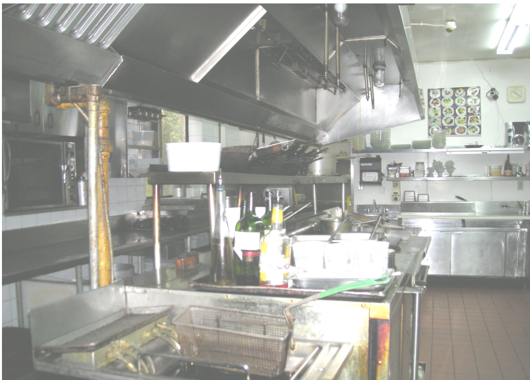
Commercial Cooking Equipment With Standard Hood And Duct, Filters Are Out Of The Hood For Cleaning, Standard Listed Lights- Note The Extinguishing System Nozzles Pointing Down To Protect Equipment.
