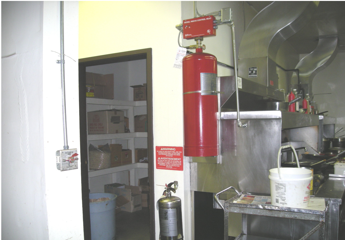
Extinguishing System Bottle Which Holds The Extinguishing Agent, “K” Type Extinguisher And Manual Pull Station.
