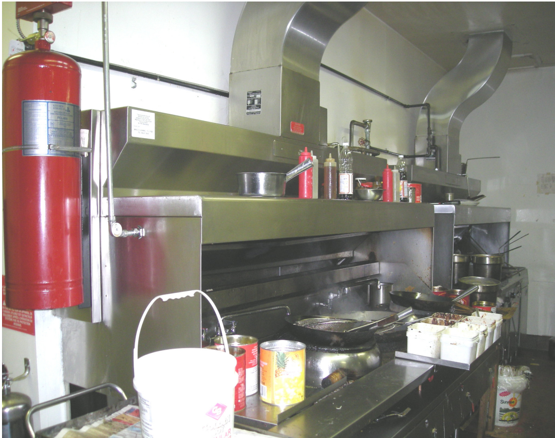
Typical Commercial Cooking Set Up-Cooking Appliances, Hood And Duct Work And Extinguishing System.
